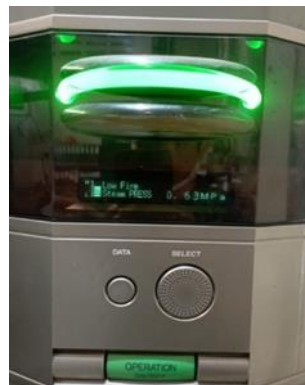
Gambar 6. Pengecekan pressure boiler .
